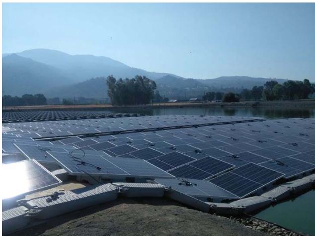
Floating solar array—Lake County
