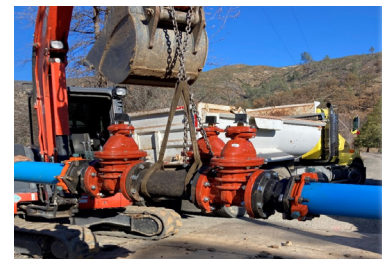
Project Managed by LSDA Administration; Quail Trail Water Line Replacement: Installation of 3-valve assembly at the intersection of Spring Valley Road and Quail Trail.
