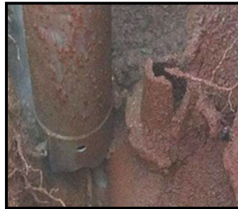
Damage from root intrusion.
