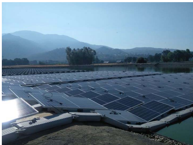
Floating solar array—Lake County
